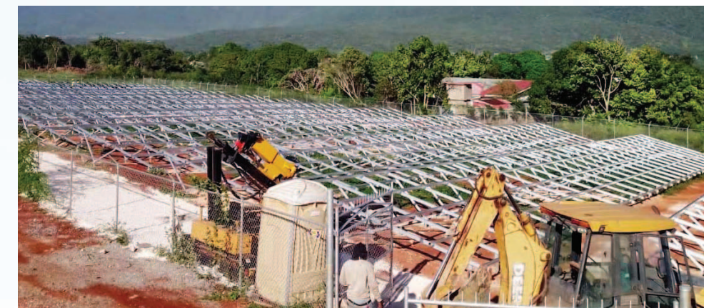
Outlay of solar panels being installed in respect of the Essex Valley Agriculture Development Project at the site in Prospect, St. Elizabeth.
